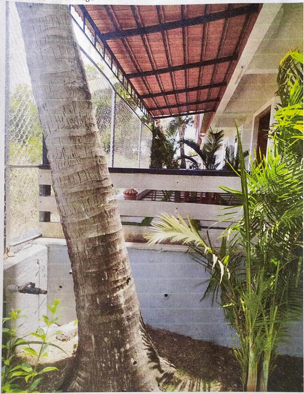
No 2: Extensions to the ground floor into western setbacks upto boundary sy.no55/3, Colva village
